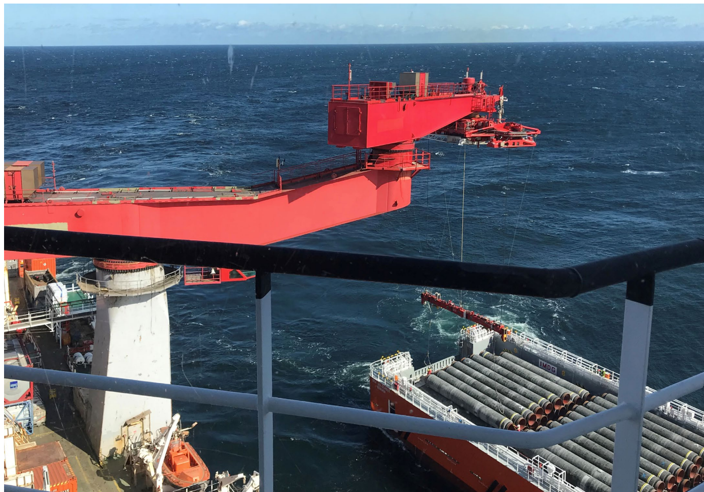
Allseas' deep sea pipe laying ship Solitaire lays pipes for Nord Stream 2 pipeline in the Baltic Sea September 13, 2019. Picture taken. Taken on September 13, 2019. Photo by Stine Jacobsen/REUTERS https://tinyurl.com/y46y2pu4
